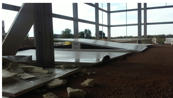
Figure 1. Cladding failure; Source: Photo taken by company Frigomex, in September 2017, Sremska Mitrovica, Serbia.
