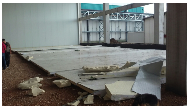
Figure 2. Panel failure: Delaminated metal facing; Source: Photo taken by company Frigomex, in September 2017, Sremska Mitrovica, Serbia.
