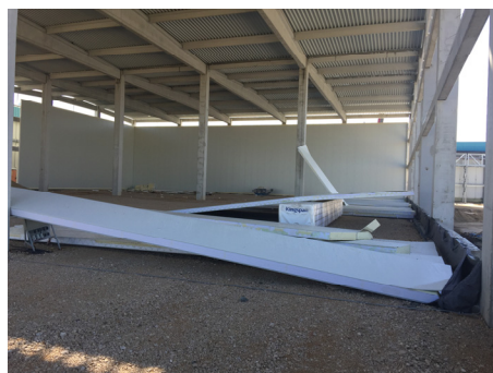
Figure 3. Pull-through failure of fastenings; Source: Photo taken by company Frigomex, in September 2017, Sremska Mitrovica, Serbia.
