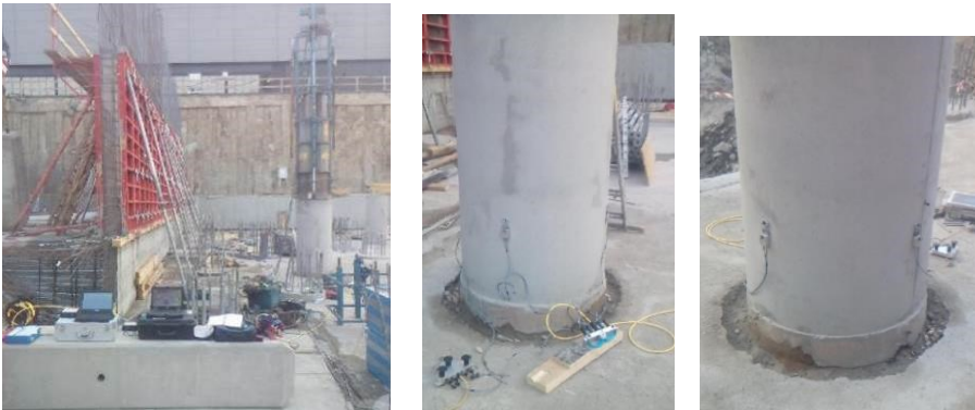
Figure 7. Pile bearing capacity testing using the DLT with two equipment (simultaneous acquisition and signal processing - 4 sensors and 8 signals)
