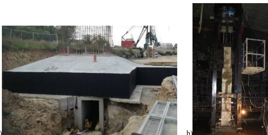
Figure 7. SLT - reactive system: a) viaducts for fast railways in Čortanovci, Serbia (reactive system formed from reinforced concrete foot – top foundation slab for piles), b) MFC Ušće business centre in Serbia (reactive system formed by presses pushing against the supporting structure)
