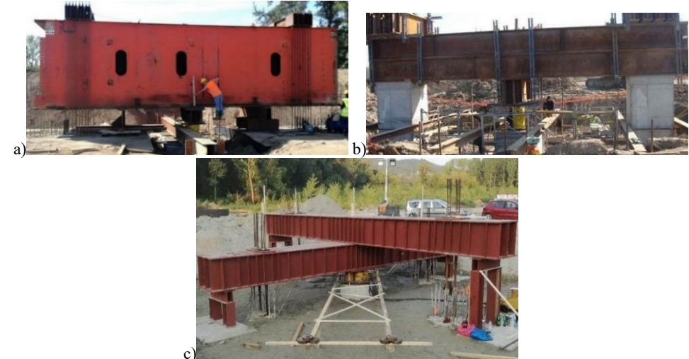
Figure 6. SLT - reactive system: a) bridge on corridor XI (Surčin-Obrenovac) in Serbia (reactive system formed from welded steel beam and four reinforced concrete piles), b) fly ash silo at TE Kostolac B in Serbia (reactive system formed of additionally reinforced dual steel beams and two reinforced concrete piles), c) fast railway viaducts in Čortanovci, Serbia (reactive system formed of double-crossed steel sections and four reinforced concrete piles)
