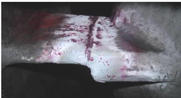
d) cracks and porosity
