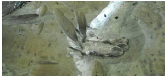
b) place of leakage and porosity
