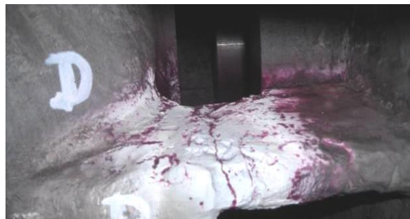
e) through cracks and porosity
