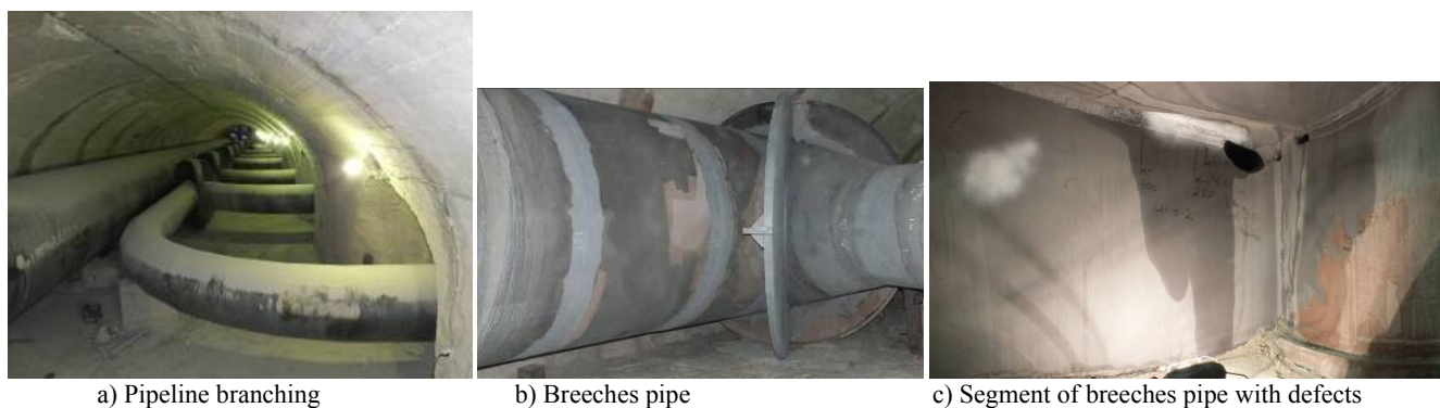
Figure 4. Pipeline III with defects in parent material and welded joints.
