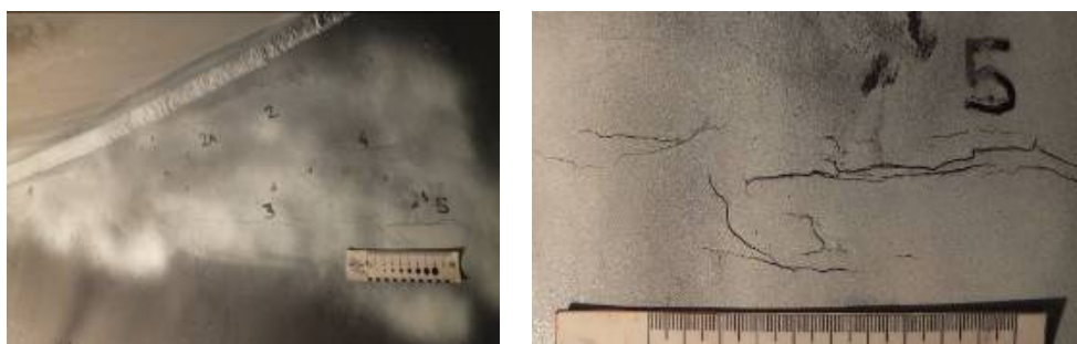
Figure 7. Cracks at the surface of parent material of the anchor of breeches pipe no.1.
