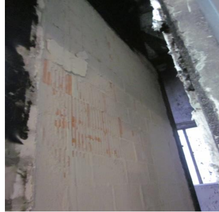
Figure 11. Exposed fire side of a wall at the end of test
