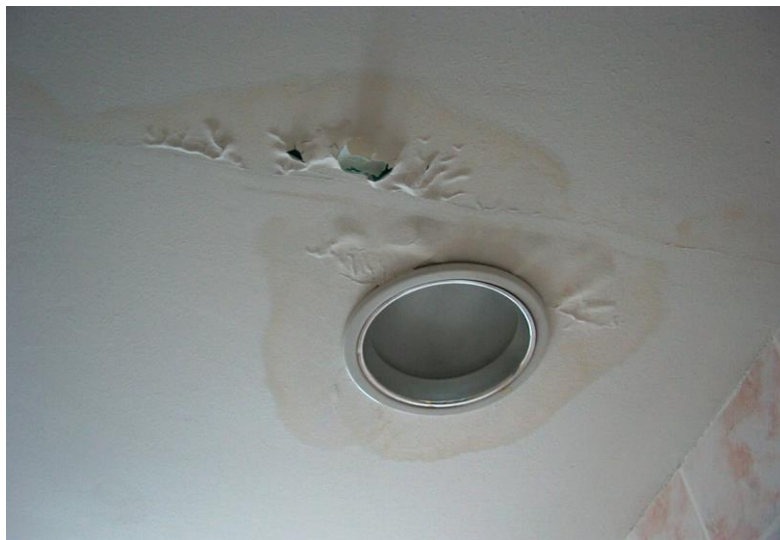
Figure 10. Leaking of the ceiling around the lighting fixture. July 2004.
