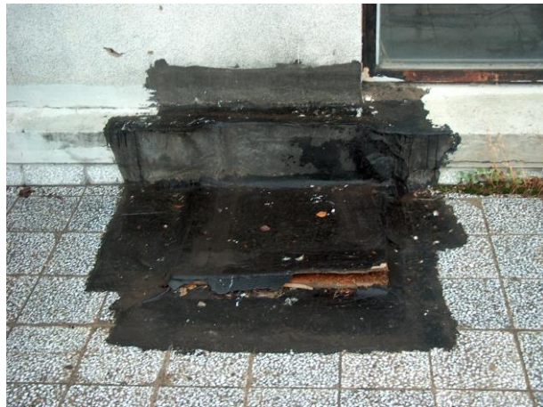
Figure 7. Opening on the roof closed off with the plywood panel. Waterproofing damaged in one part. July 2004.
