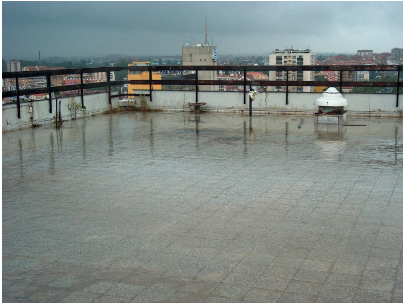
Figure 6. A view of the flooded roof terrace and unplanned roof plants near the attics. July 2004.
