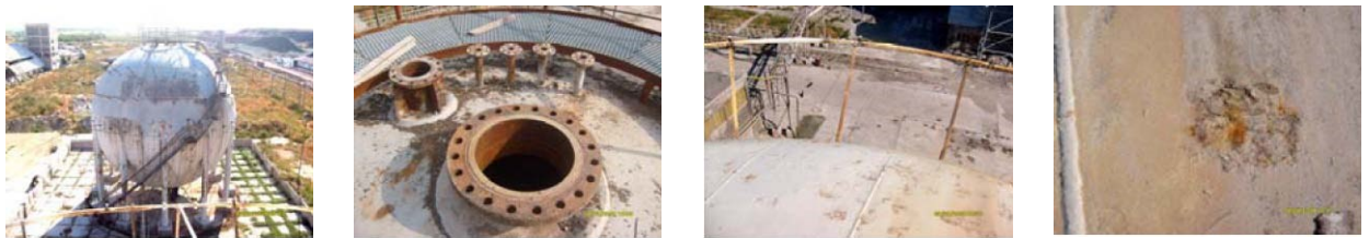
Fig. 5. Examples of corrosion damage to the construction of a spherical tank (Aleksić V., 2009 /5/)
