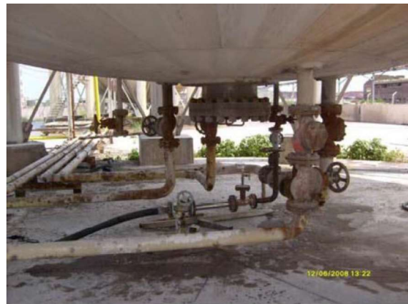
b) pipelines for streaming and filling
