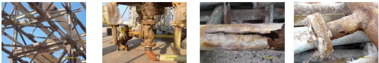
Figure 2. Examples of corrosion damage to pipeline steel structures [1, 2]
