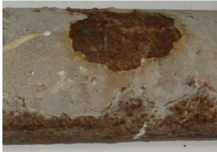
Corrosion damaged pipe
