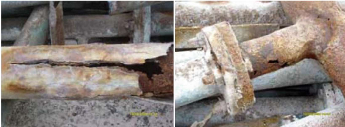
Fig. 1. Examples of corrosion damage to steel support structures of pipelines [1, 2]
