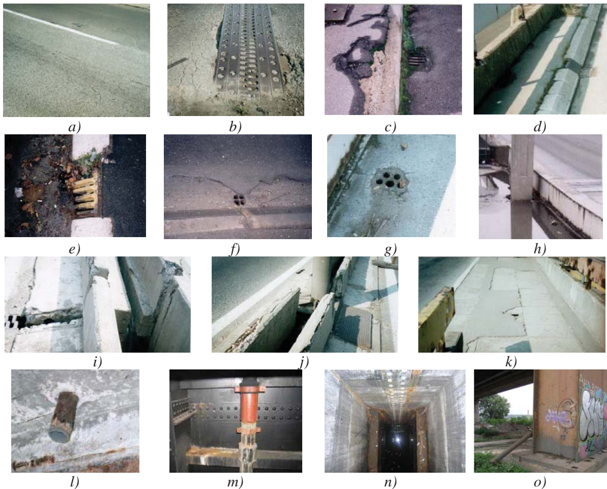
Figure 4. Degradation of the drainage system of bridges and materials around it [10, 11]
