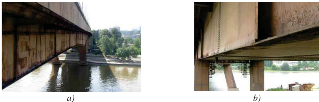
Figure 7. Degradation of steel structural parts. Examples of corrosion damage of steel bridges [11]
